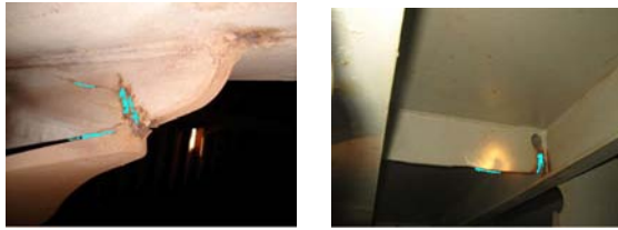
Fig. 12. Cracks detected by GPCD.
